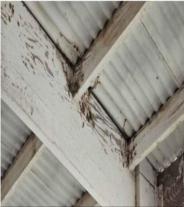
13. Remnants of swallow nests on the underside of the shaded picnic tables on the south side of the boat ramp. This part of the shade structure overhangs the water and is the highest off the ground.
