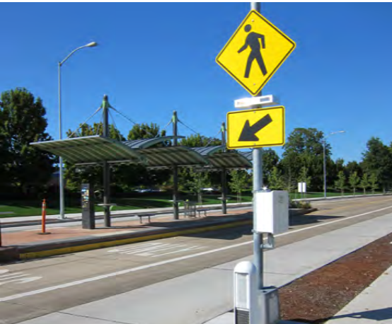
Rectangular Rapid Flashing Beacon (RRFB)
