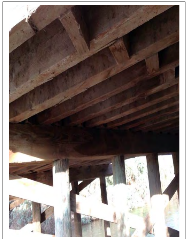
8. From the south Bank of the New River the picture taken is from the midsection of the bridge looking south, no nesting birds or 77 bats were observed.
